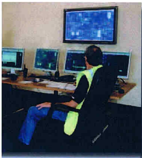
Above: Commissioning underway in a temporary control room. The plant uses a Raytek kiln scanner
