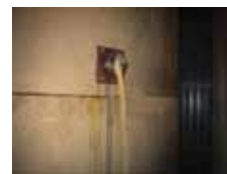
Tube is removed to reveal build-up has been cleared and product is aerated and once again free flowing.
